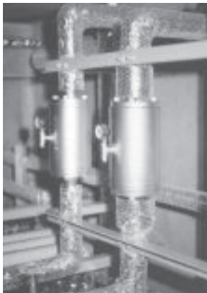
Installation in riser for lift pump
