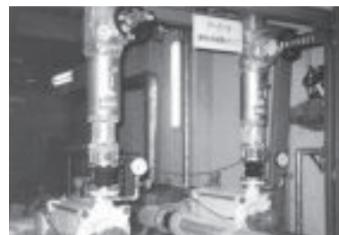
Installation in riser
